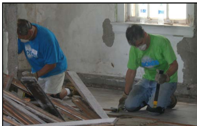
Volunteers from Lubrizol Corp. remove the floor from a Kinship Village building in preparation for renovation.
