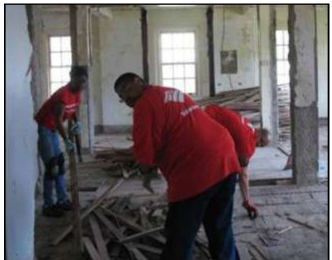
Bank of America employees remove floorboards from Building 6 of Kinship Village on June 9.
